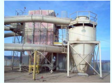
Dust collector retrofitted due to moisture and filter clogging problems
